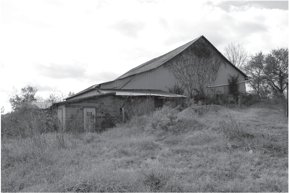
Supported by massive hewn timbers now hidden by modern siding and additions, the barn where Anne Bunnell ended her life in 1825 stands today in Lebanon, Ohio, on the disputed property Benjamin Scudder deeded to his daughter and son-in-law in 1801. Photograph by Nate Byrum.
